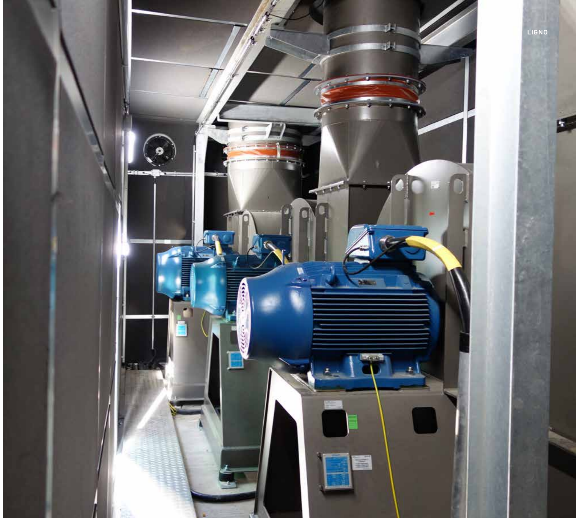
The Derix Group relies on ventilation systems from Scheuch LIGNO at its plant in Westerkappeln, Germany.
