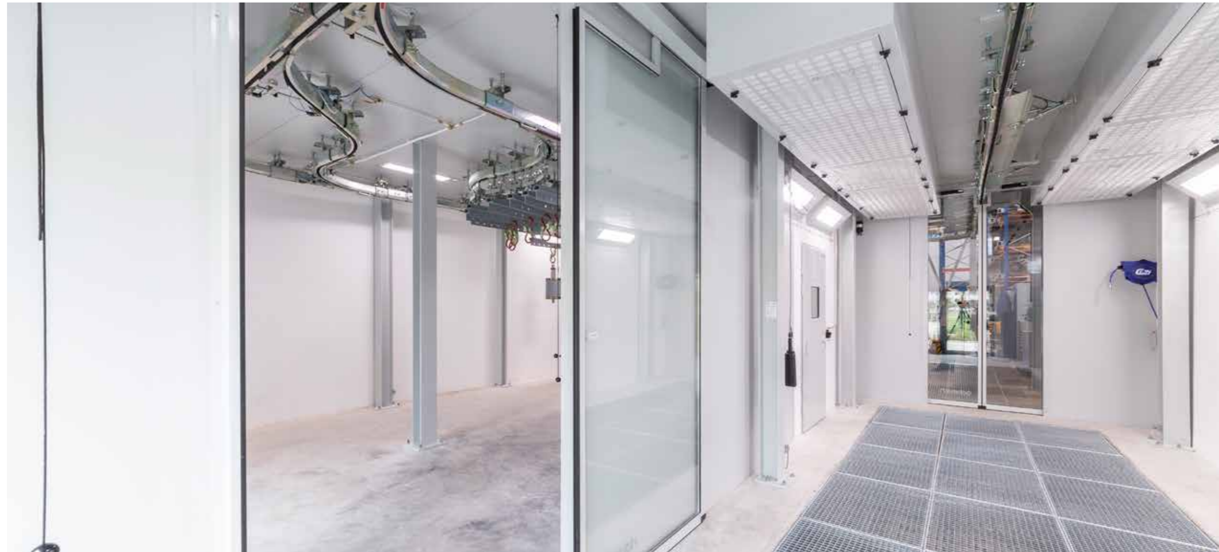
New spray booths for perfect surfaces.
